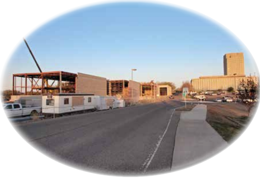
The April 11, 2012 photograph above shows the construction progress on the three new galleries of the North Dakota Heritage Center. Shown below is the architect's rendering of those galleries.
